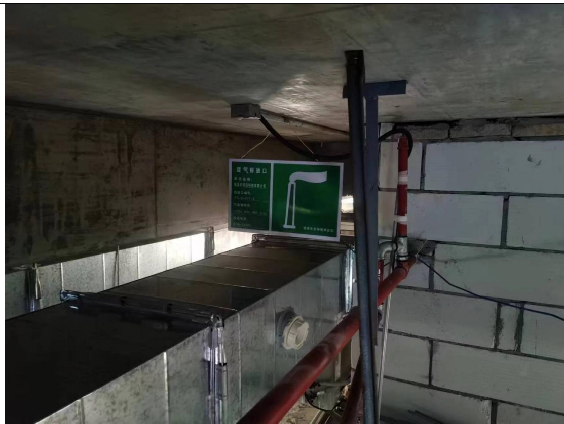
FQ-6-277-2 废气排放口标志牌
