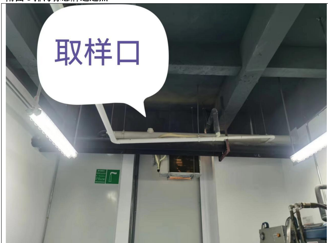
FQ-6-277-1 废气排放口标志牌
