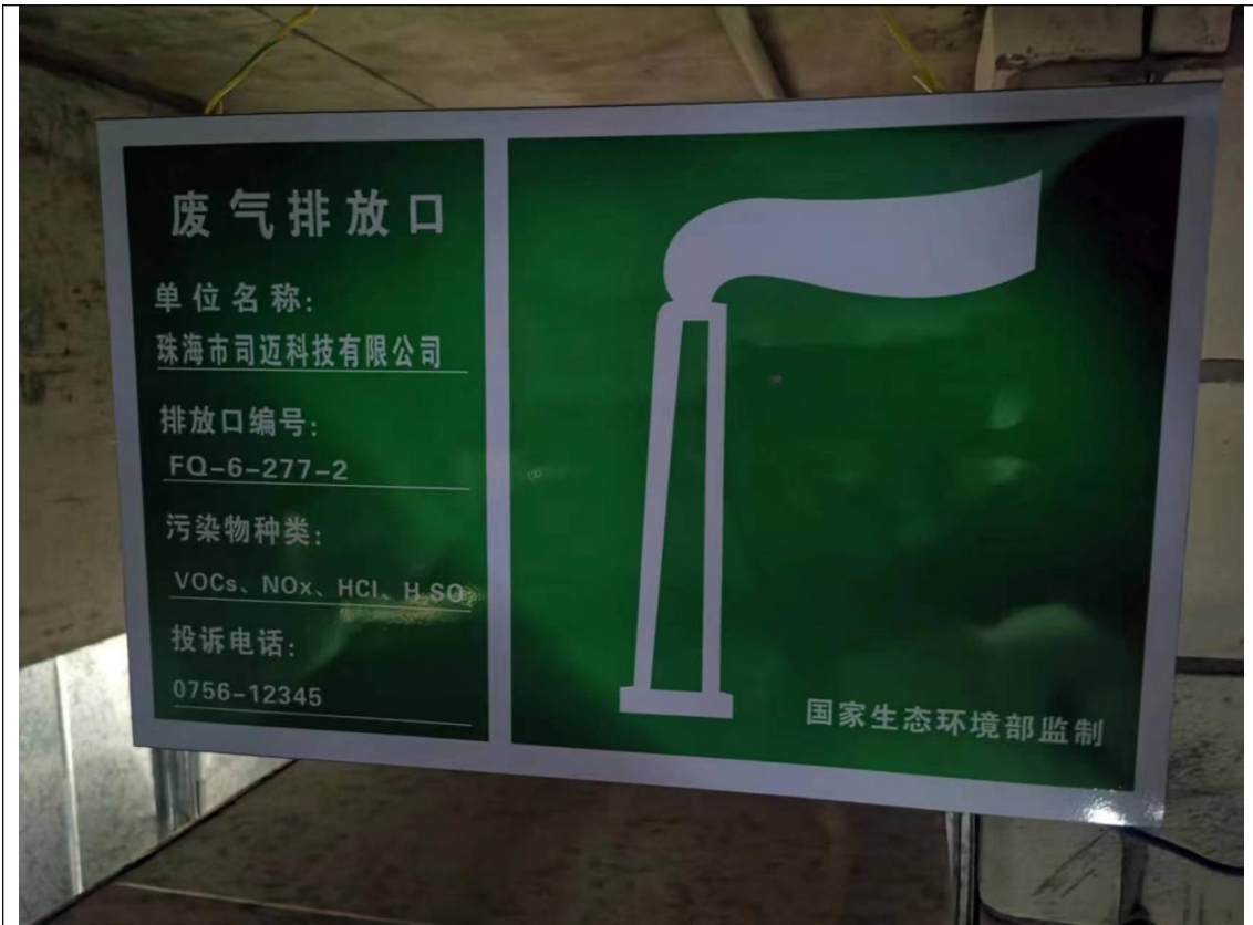
FQ-6-277-2 废气排放口标志牌
